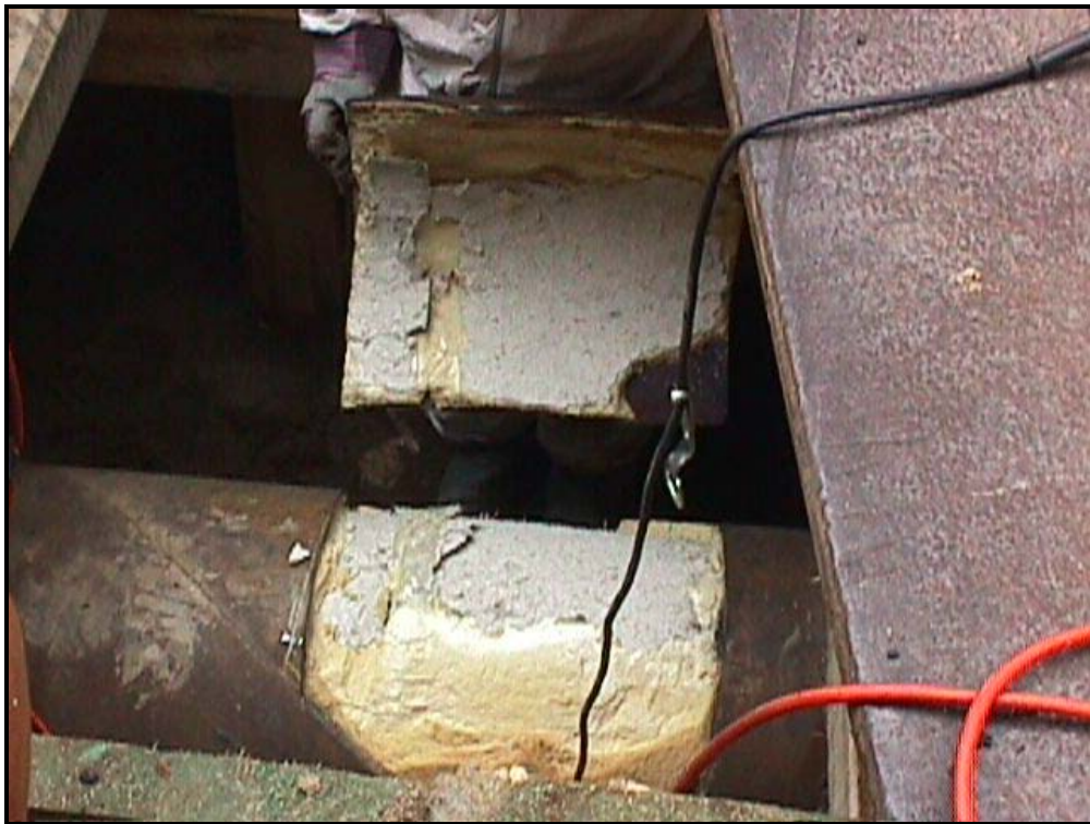
The casing is removed to reveal that ConduFill® (gold) had indeed filled the entire void while compressing and encapsulating the existing asbestos insulation (grey).
