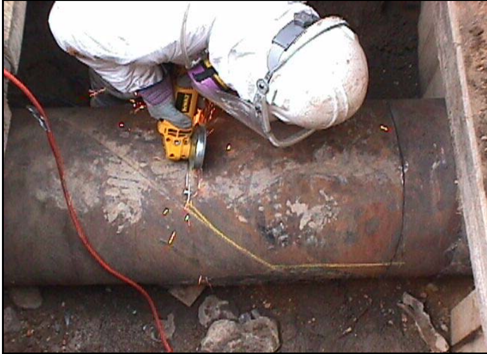
The outer steel casing is carefully cut with a grinder by a Con Edison employee.
