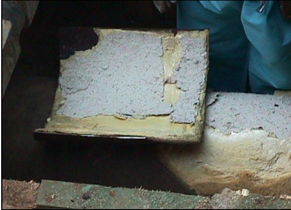
A closer look of the opened steel casing reveals that the ConduFill ® insulation adhered to the outer casing when it was removed. The existing asbestos insulation (grey) also adhered to the inner layer of ConduFill ® .
