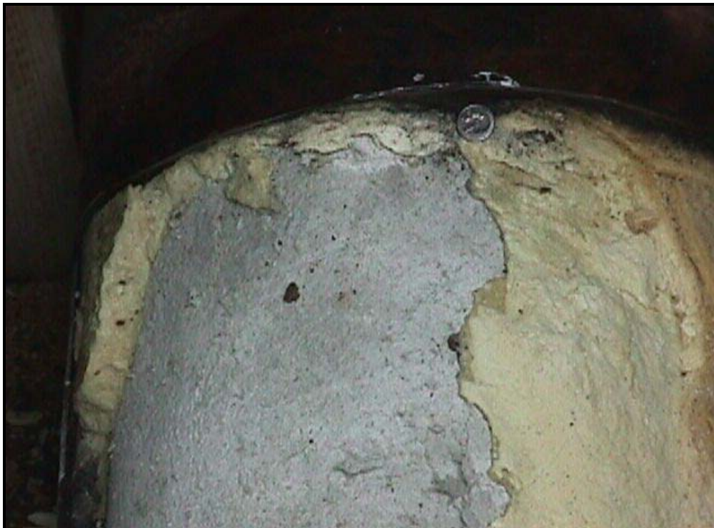
A closer look at the section of ConduFill ® that was manually peeled away from the existing asbestos insulation.
