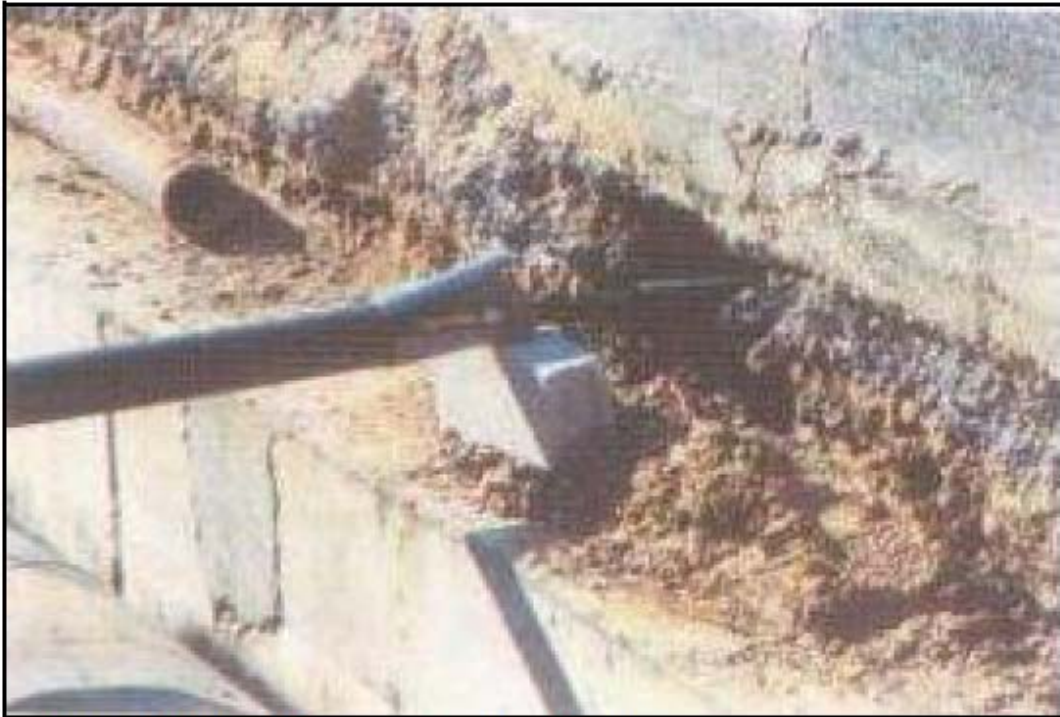
Fig. D - Site leak area locator above the trench opening
