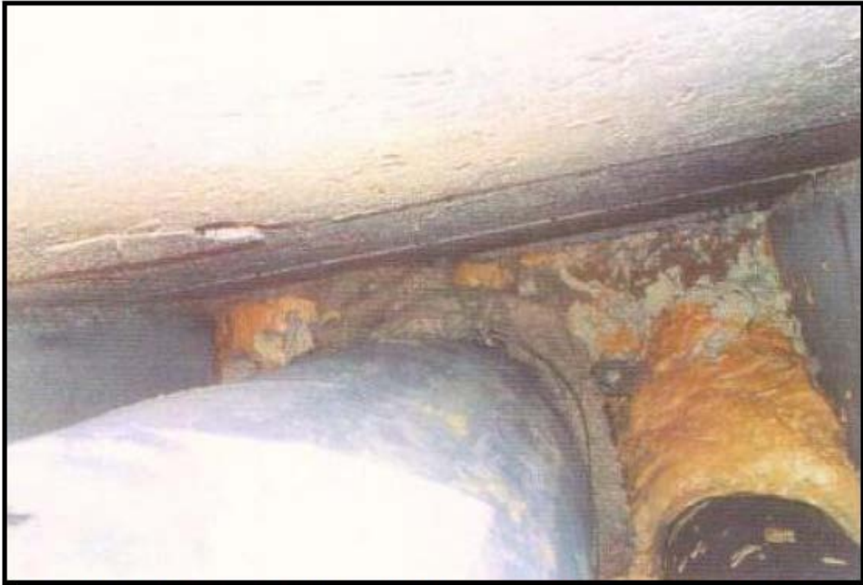
Fig. E - Void in between two ConduFill SM areas (only one end can be seen)
